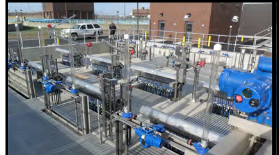
Bergen Point Wastewater Treatment Plant
